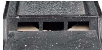
top view of completed speaker installation.
